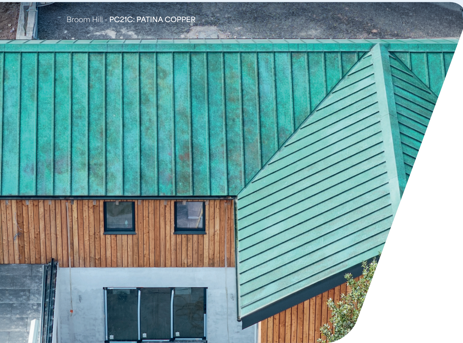
Cover image Tramm Inn - PC211: RUST
